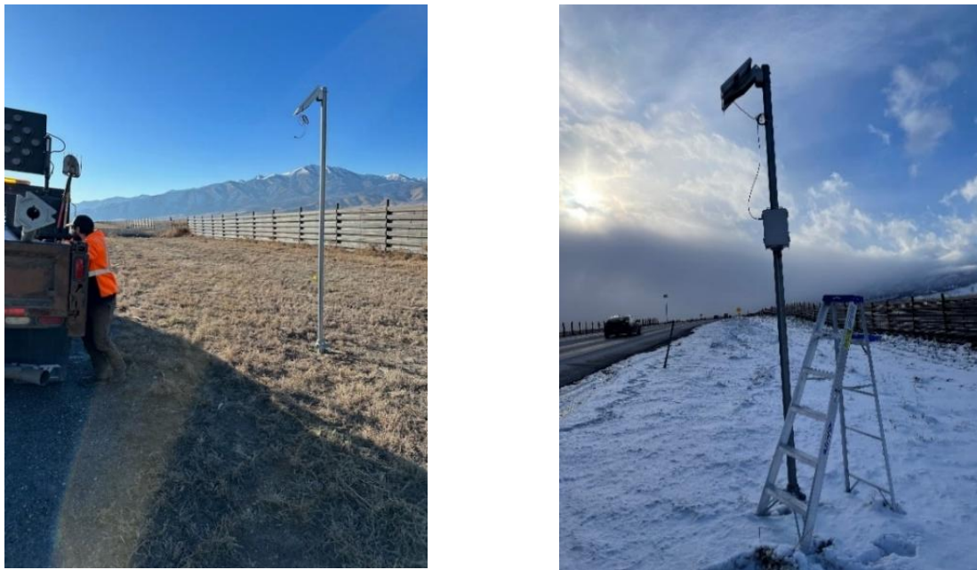
Figure 5. Posts and solar panels installed by UDOT and Stalker, left, and Stalker Traffic Data Collectors with solar panels, right. Photo credits: UDOT and P. Cramer.
