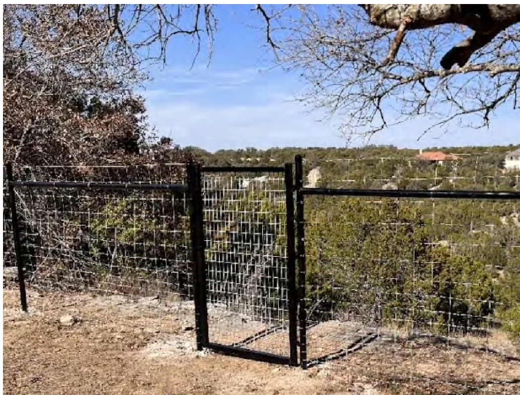
Wildlife Fencing with Gate and Metal Post
